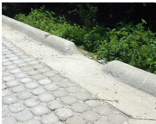
Figure 1117-A: Cuts in the continuous curb allow for stormwater to be directed into landscaped areas.
